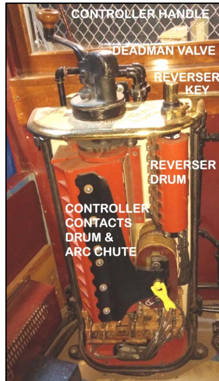
Controller with cover removed
