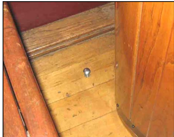
Water foot-valve on floor near each controller.
